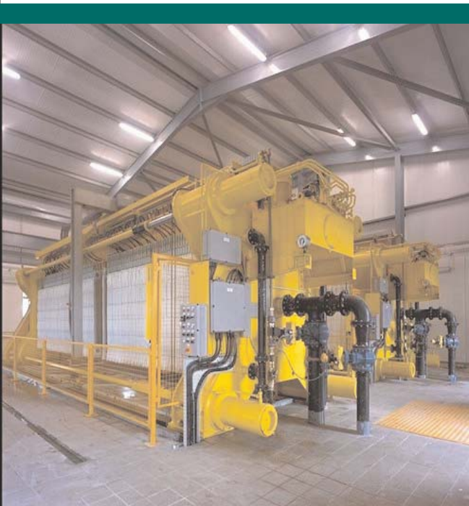
Membrane Type Sludge Presses
