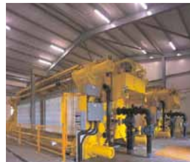
Membrane Type Sludge Presses
